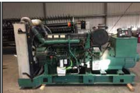
2006 Volvo 550 KW Gen Set 480 Volt, recent engine repairs $48,900
